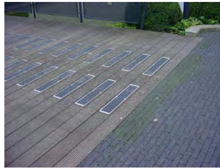
Antislip houten toegangspad. © Inter
