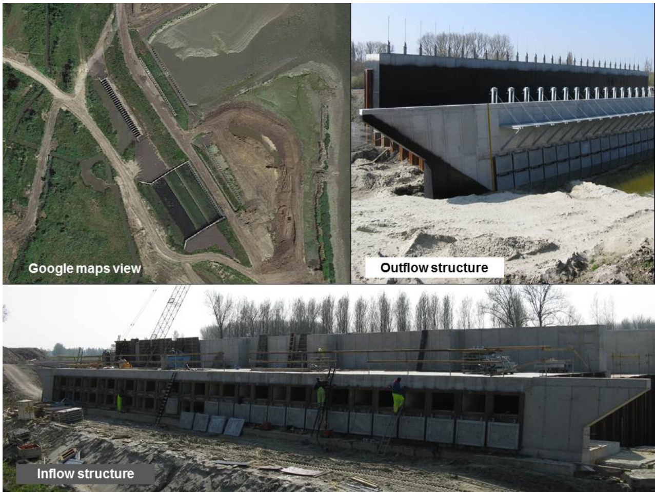
Figure 23 – Pictures of the in- and outlet structure under construction of the Kruibeekse polder.
