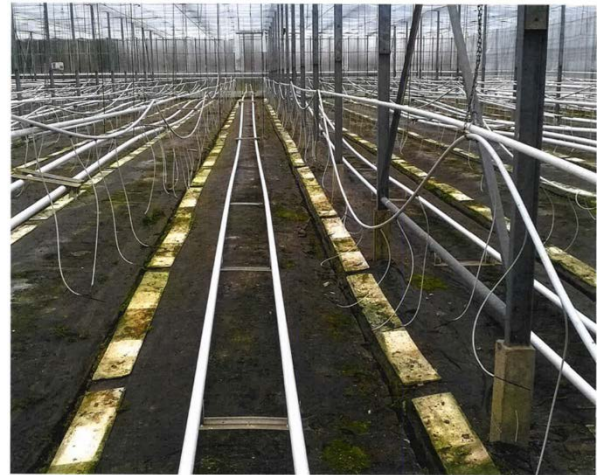
Photo View of the greenhouse without plants, the plastic film is worn. We told the horticulturist to replace the film and also to renew the connections on the drainage pipes.
