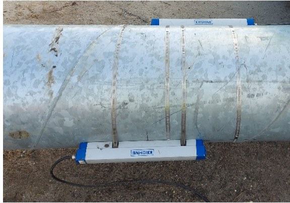
Figure 15 – Set-up Khrono Optisonic discharge measurement
