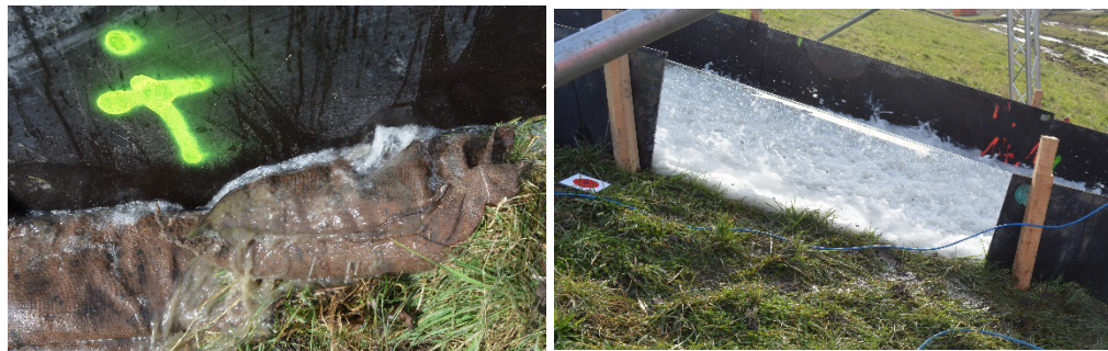
Figure 10 –Leakages (left) and transparent side boarding (right)
