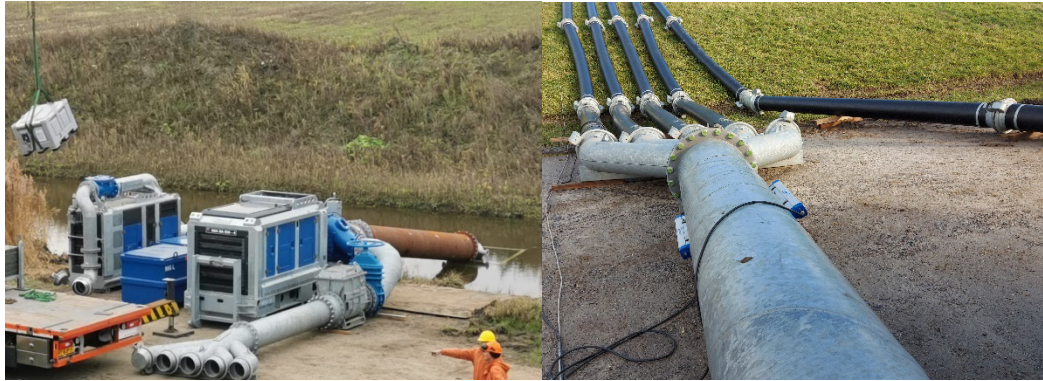
Figure 4 – Setup with two individual BBA pumps and parallel feeder lines.
